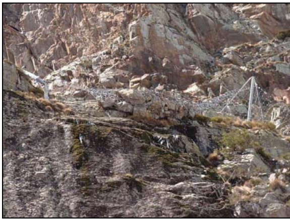
Figure 21: Picture showing mass stopped by one of the upper barriers in April 2003 event.
