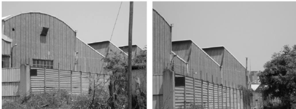
Figure 5: Photographs of the building affected by thermal deformation. Note the metallic structure of the building.
