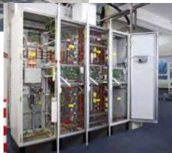
battery/cells testing lab
